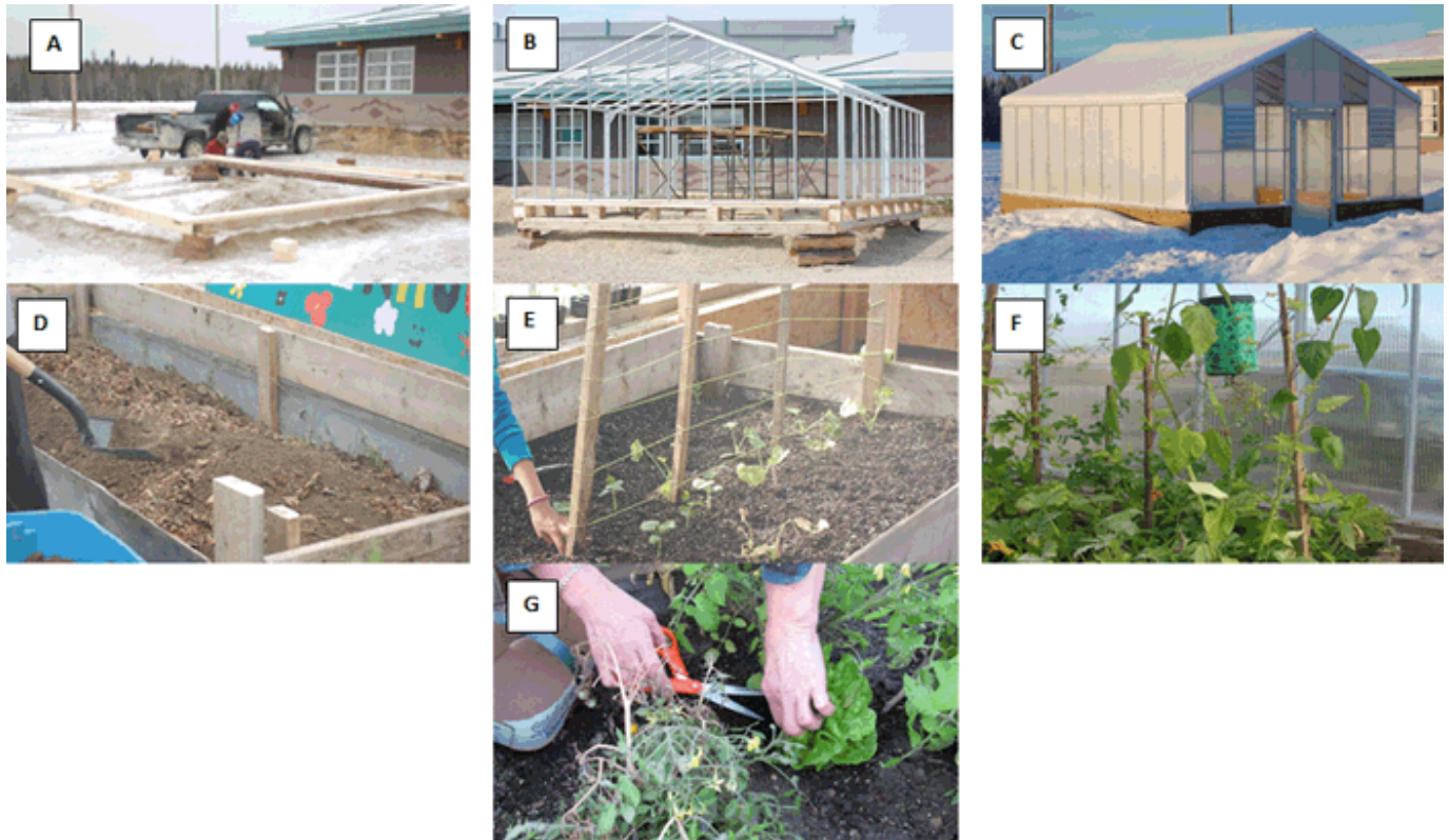
Figure 2: From construction to harvest. (A) 21 November 2009: Following the arrival of the greenhouse pieces, a few teachers and community members began to construct the foundation for the greenhouse out of wood from the local sawmill. Community members felt it was important to have the foundation initiated and to let it sit over the winter and spring thaw to make sure that it would not shift through the seasons. (B) 16 June 2010: Greenhouse construction in progress during the following summer of 2010. (C) 11 January 2011: The greenhouse was built and sat under a blanket of snow, waiting for spring to arrive. (D) 25 June 2011: Inside the greenhouse, raised garden beds were built out of wood and filled with dirt. (E) 29 July 2011: A young girl helped to meticulously plant seeds in one of the raised beds in the greenhouse. (F) 2 October 2011: Vegetable plants, even sunflowers, thriving in one of the raised beds inside the greenhouse. Beans, peas, carrots, squash, tomatoes, various types of lettuce and a few flowers were planted and grown in the greenhouse. (G) 5 October 2011: Harvesting a head of lettuce to make a salad for dinner.
